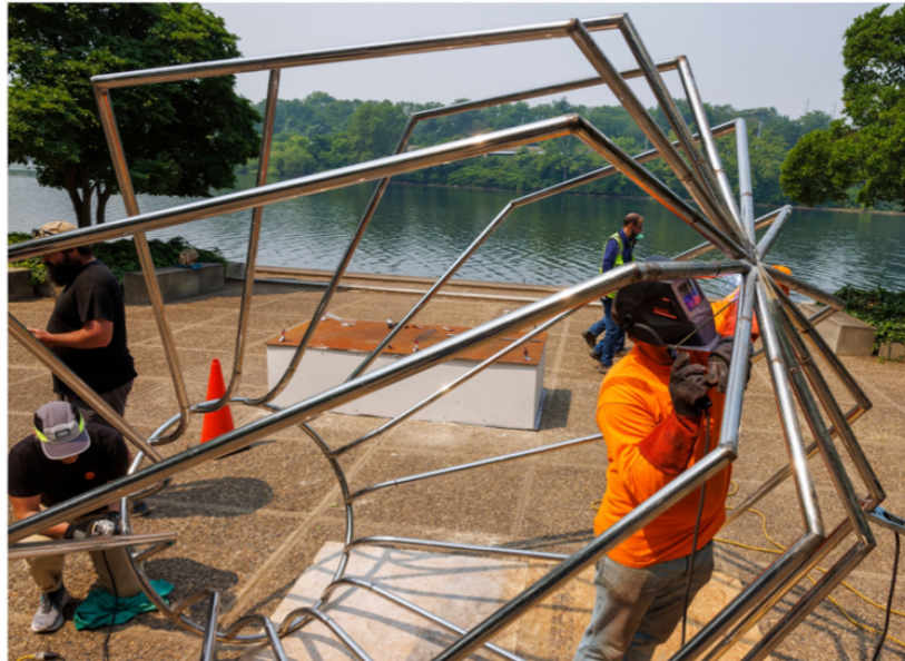
Travis Johnson with Atelier Fine Art Services welds "Vessel 10" from Maren Hassinger's "Steel Bodies" exhibit along Kelly Drive. Alejandro A. Alvarez / Staff Photographer
