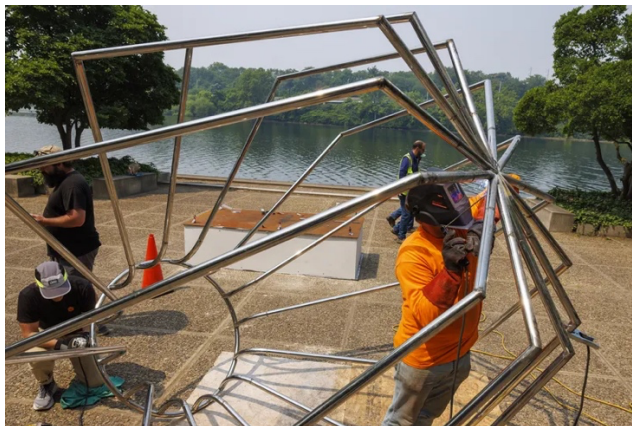
Travis Johnson with Atelier Fine Art Services welding the piece titled Vessel 10 from Maren Hassinger's "Steel Bodies" exhibit at the Ellen Phillips Samuel Memorial on Kelly Drive. Photographs from installation on Wednesday, June 7, 2023. ... Read more Alejandro A. Alvarez / Staff Photographer
